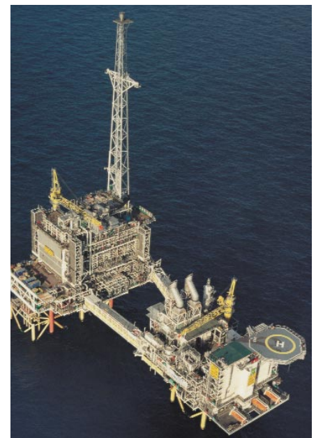
Sulfate reduction system installed on BP Amoco © ETAP
